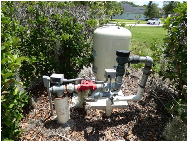
Well and Pressure Tank
