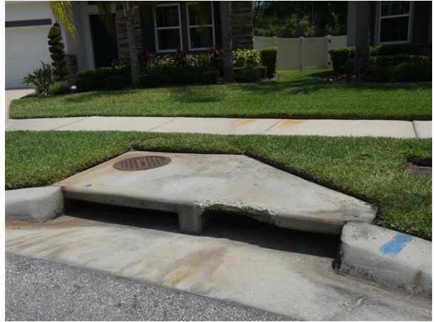
Stormwater Drainage Curb Inlet
