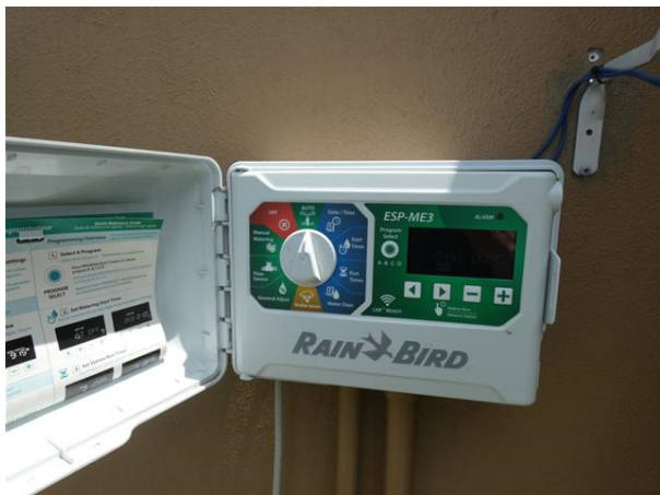
Irrigation System Controller
